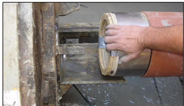
Fig 6: 8-inch Jacking Pipe being installed with a steel casing. A stack of wood rings was used in lieu of a pipe adapter push ring.
