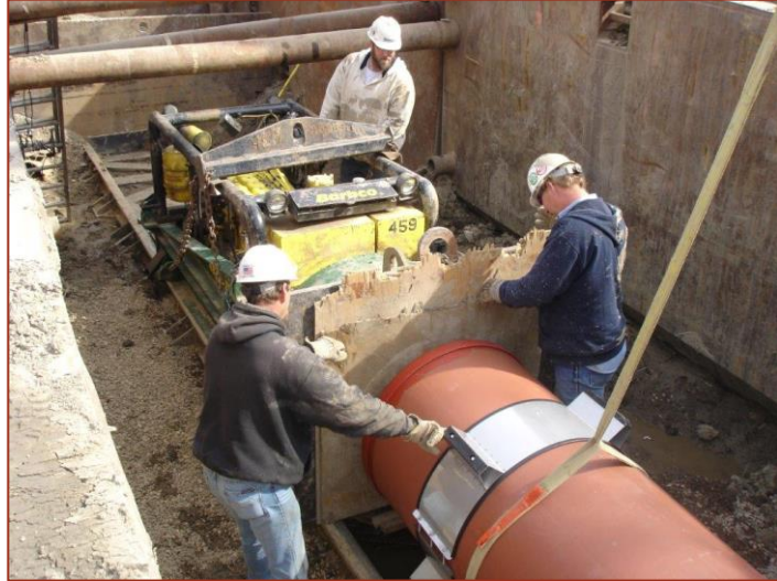
Fig 1: 30-inch Bell and Spigot pipe being pushed with a Horizontal Auger Bore Machine via the spigot end.
