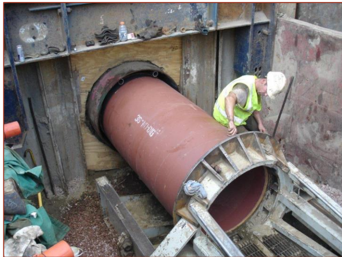
Fig 4: 36-inch Vitrified Clay Jacking Pipe installed directly on the invert of a 48-inch steel casing.
