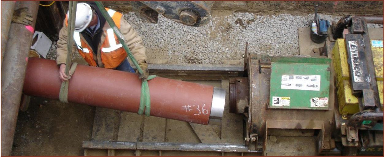
Fig 5: 12-inch Vitrified Clay Jacking pipe being installed via a Horizontal Auger Boring Machine.
