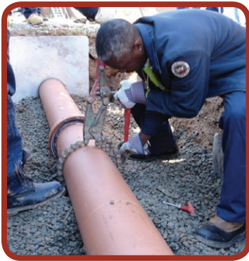
Figure 27: Cutting out a section of main line to insert a factory made, plain-end wye fitting.
