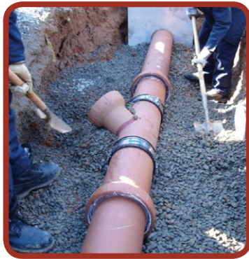
Figure 28: Wye fitting for lateral service connection to main line made using shielded rubber couplings.
