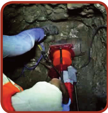
Figure 25: Core drill used to add a service to an existing pipe line.
