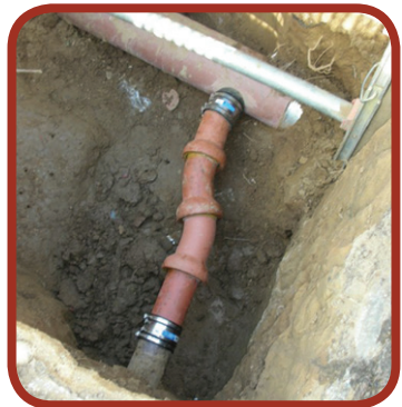
Figure 26: Hole cored in clay jacking pipe to reconnect a lateral following a pipe burst.
