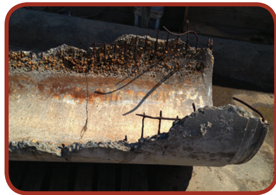
Figure 3-2: Concrete pipe degraded over years in the corrosive environment of a sanitary sewer.
