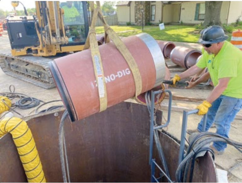
Short (1-meter) VCP-J pipe lengths make the 8-foot shafts functional
