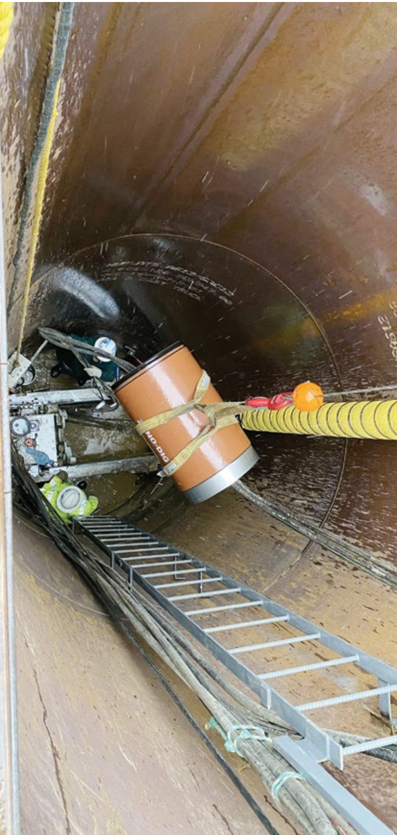
The depth needed to tie in to the existing sewer was one of the challenges that made the Pilot Tube Method of guided boring the right choice for this project
