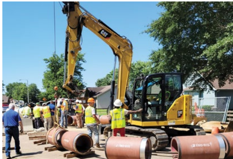
Available right of way was limited to the roadway in many parts of the project
