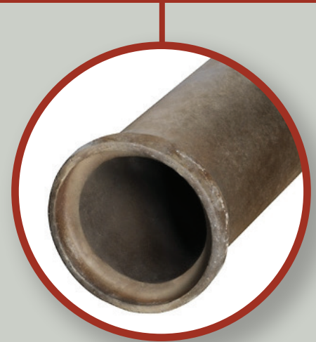
120-year old VCP pipe recently replaced to increase the capacity of the main.
