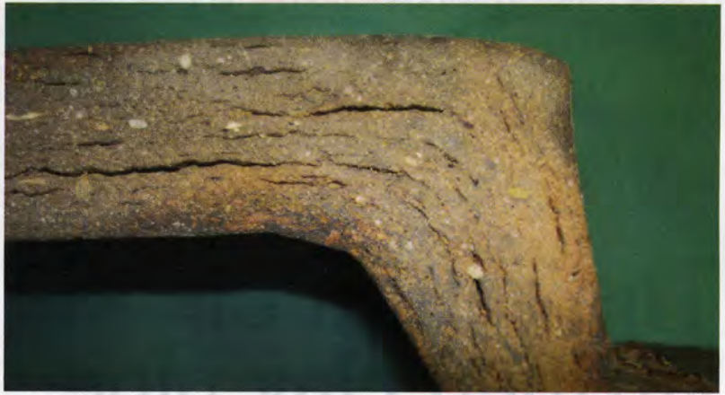
Impurities and imprecise firing methods caused voids and lamination in the terra cotta pipe placed in the late 1800s and early 1900s. Photos: National Clay Pipe Institute
