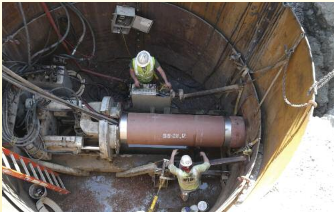
Jacking shaft installing 21-inch pipe in the final phase of the installation
