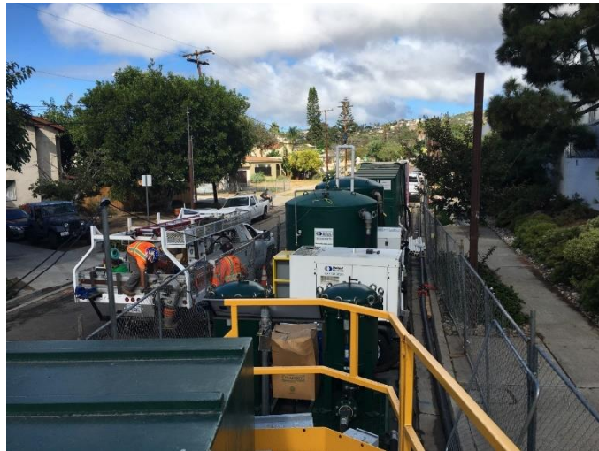
Figure 4: Onsite GAC treatment plant
