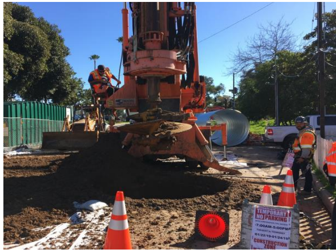
Figure 6: Riparian and tidal influence on ground waters made dewatering wells a key component of the construction plan.
