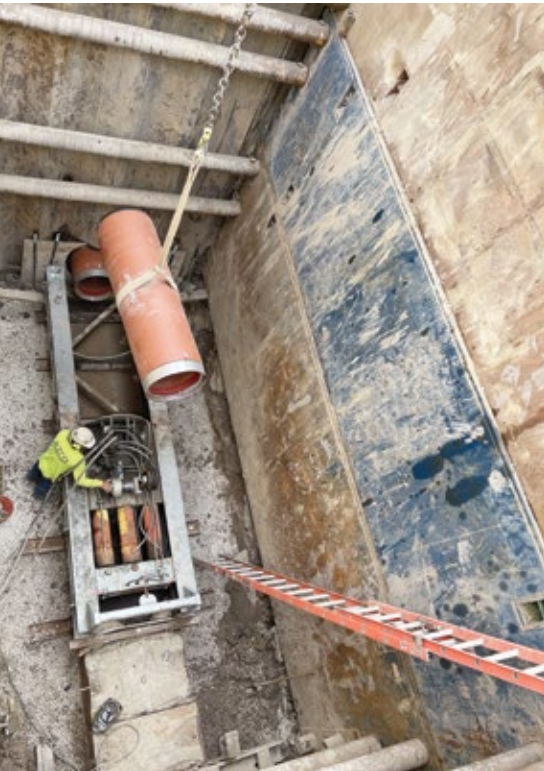
An installation depth of 25 feet was another reason that PTM was the best option for this job
