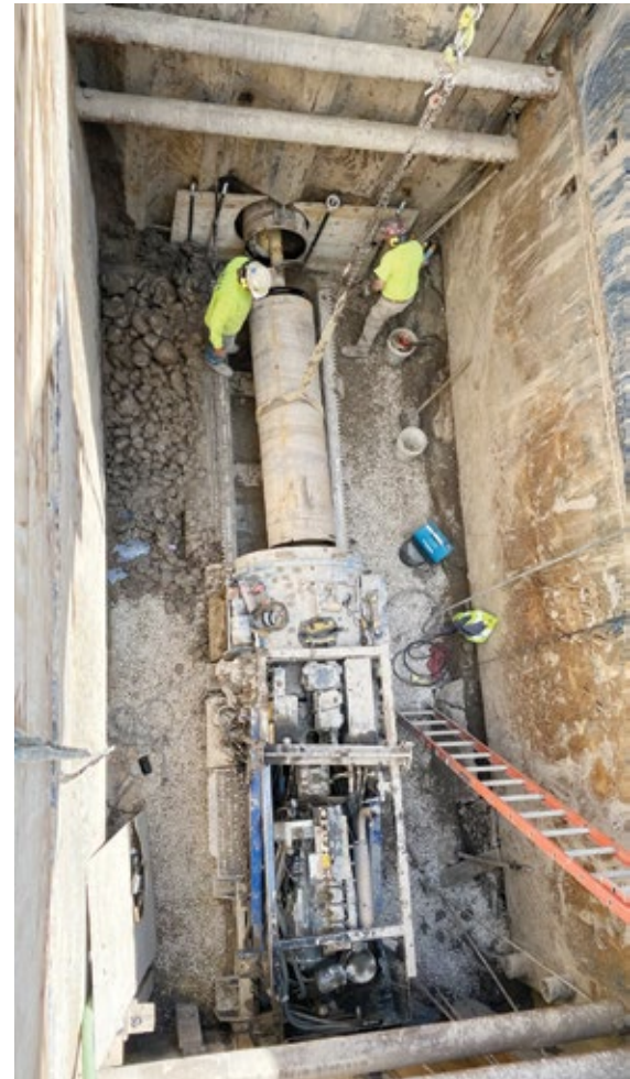
The American Augers 36-600 auger boring rig installing the 25-inch diameter by 10ft length temporary steel casings in the second step
